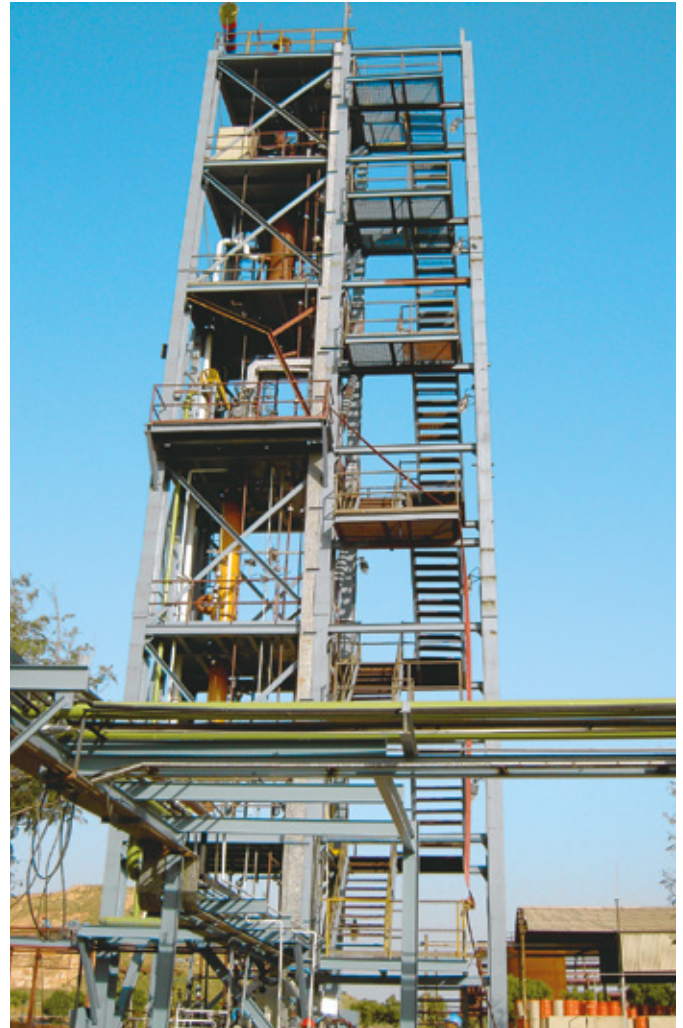
↑ Decomposition unit for processing fluorinated hydrocarbons
